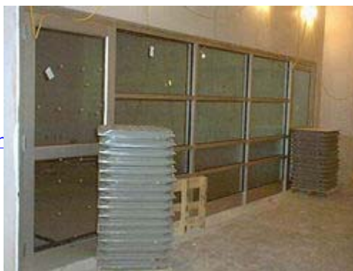
APRIL: New Engineering Room front.
