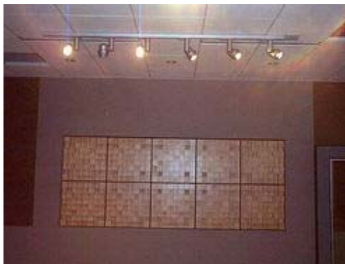
June: RPG diffusers in new Master Control Room.
